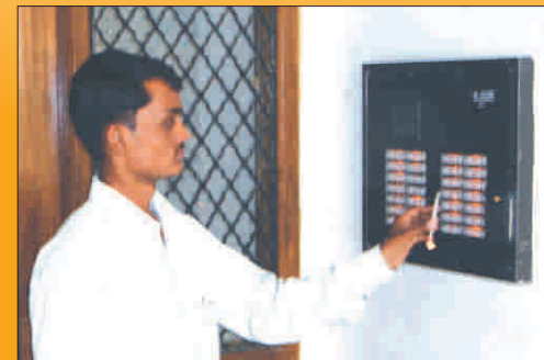
Card access security system in entrance lobby
